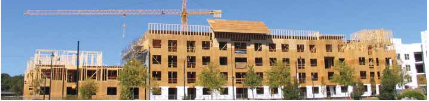
Construction staging requirements in the dense development challenged builders but one project architect, Ron Harwick, said they could not have achieved the economics and the density without using wood.
