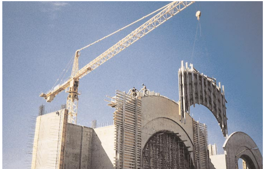
A crane hoists into place portions of the 6,800-square-foot gang form composed of APA Rated HDO plywood panels.
